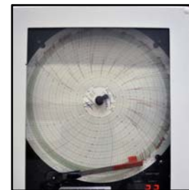
Fig. 36. Monitor temp of bulk tank
