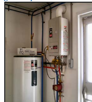
Fig. 16. Hot water tank in good repair
