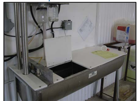
Fig. 44. Covered wash sink helps maintain temperature of wash water
