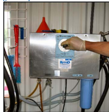
Fig. 42. Wash control box in good repair
