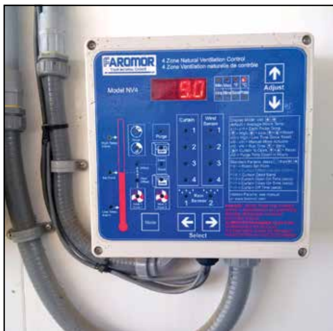
Automated Ventilation Controllers
